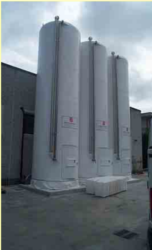
40 flour tons storage in 3 glass-fibre silos with weighing system installed to Cepagatti (PE).
