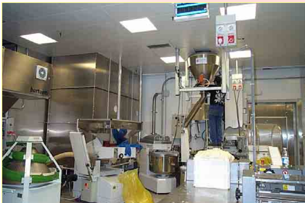
Metal silos with fluidized bed installed to Mantova
