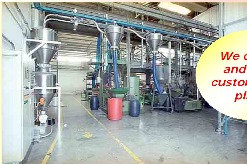
Automatic storage and dosing plant for the plastic packing production
