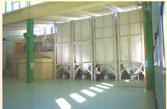
155 tons of bran storage system for the production of cous cous in 4 silos in Trevira® fabric.
