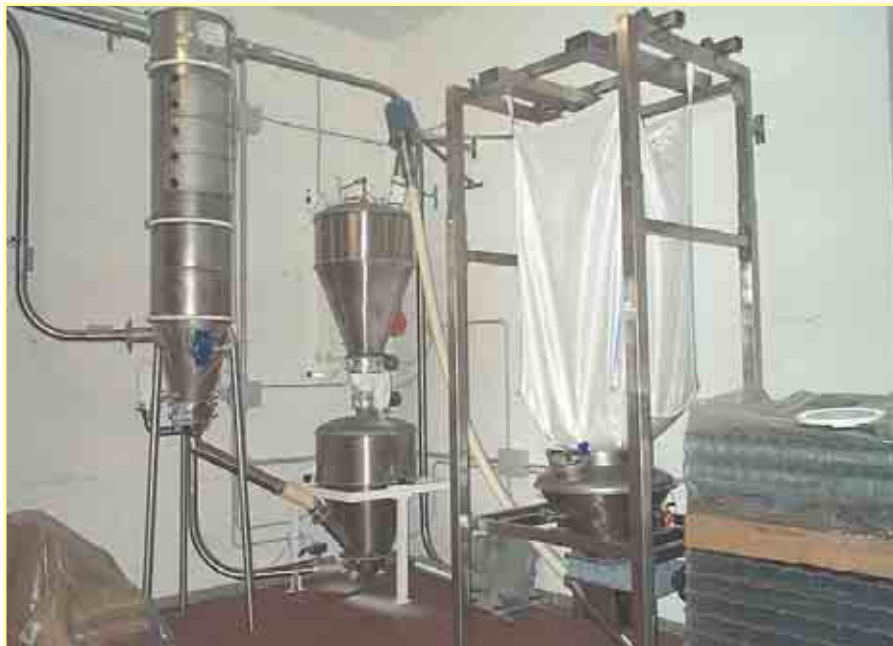
Unload big bag station for the sugar's automation installed to Lovere (SO) in a manufacturing firm of jam.
